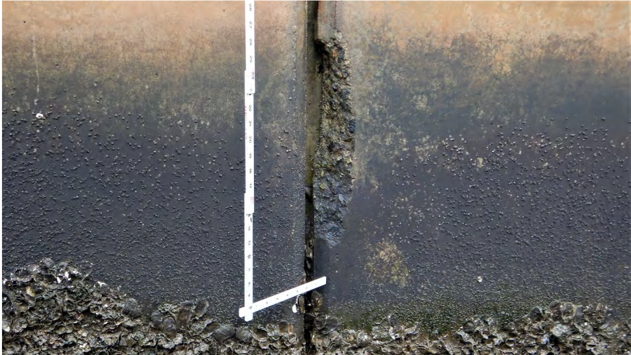
Note tongue-and-groove fit between the sheets, visible inside the spall
