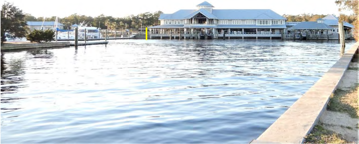
View of DPM bulkhead wall at marina inlet (foreground left and right) and end of scope limits between Ferry Terminal Building and A Dock (yellow, background center-left)
