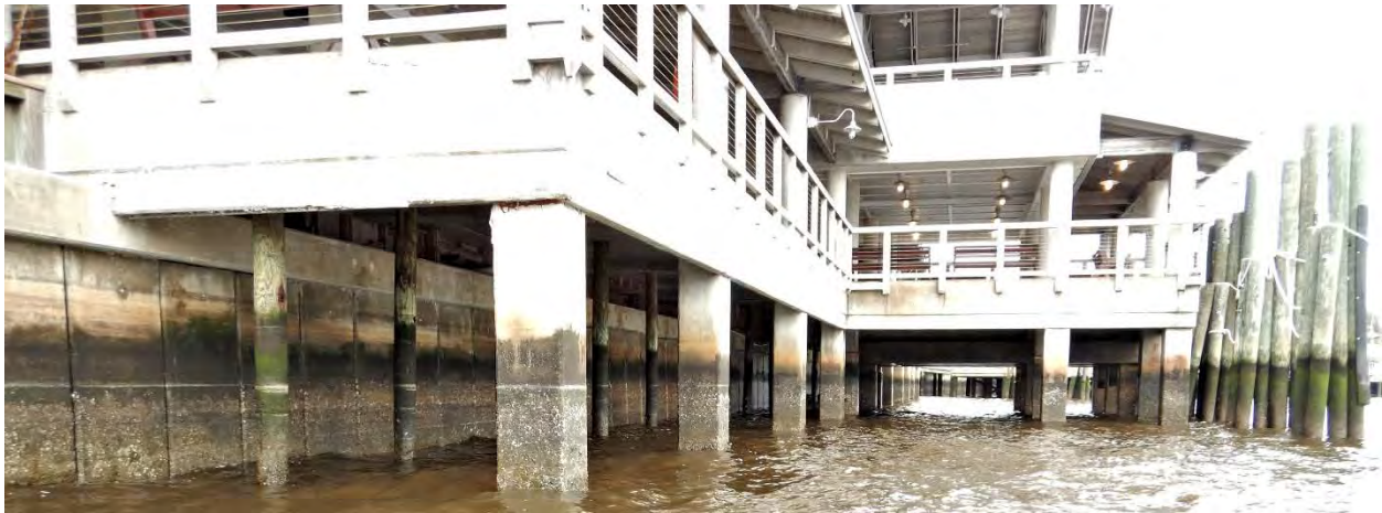
End view of concrete support piles, timber fender piles (right), and adjacent concrete bulkhead (left)
