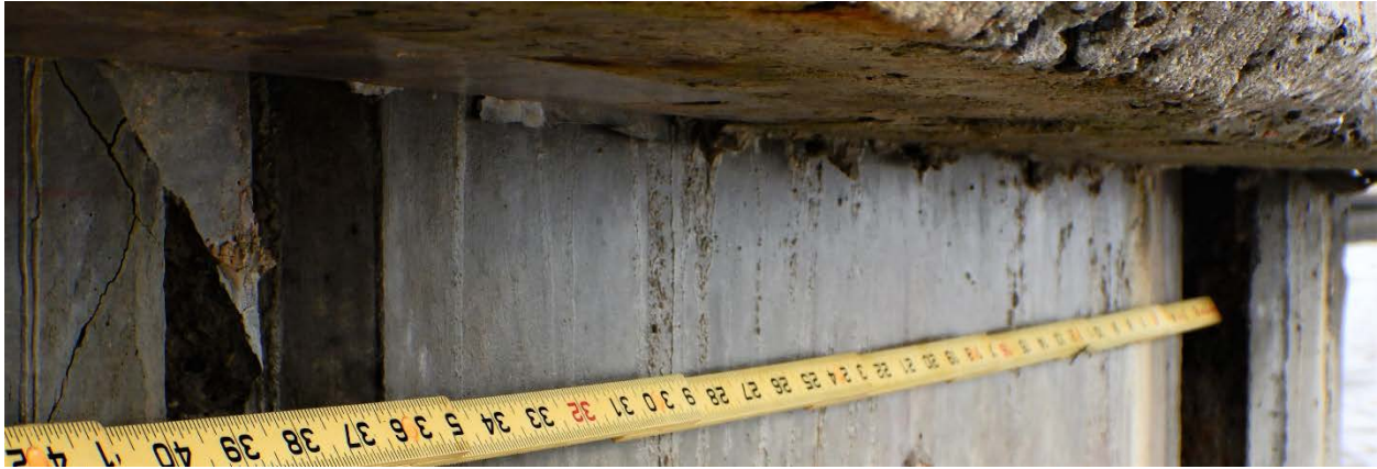
FIGURE 2-17: DISPLACED CONCRETE SHEET PILES AT BULKHEAD REPAIR SECTION
