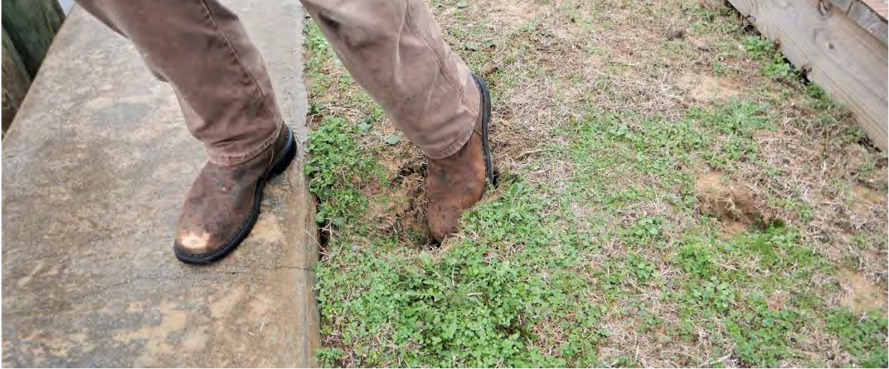
FIGURE 2-15: TYPICAL SINKHOLES BEHIND WALL
