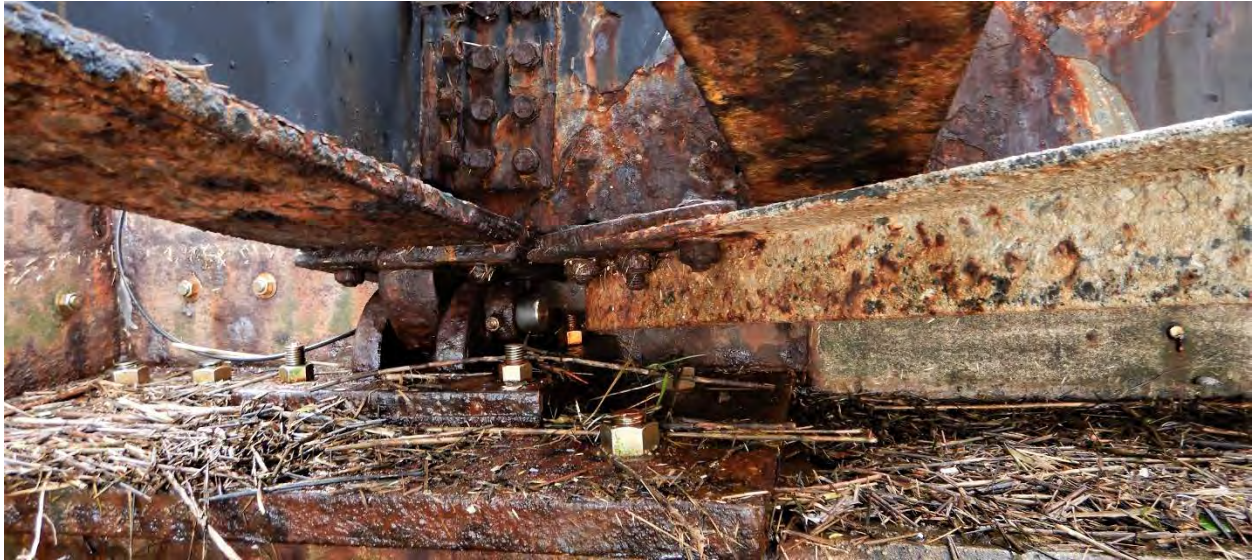
FIGURE 2-21: BHI BARGE RAMP STEEL FRAMING MODERATE CORROSION
